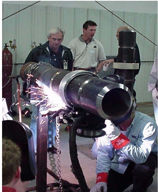
Figure 2. Live demonstration of automatic orbital welding of a fixed 5G (double up) P91 pipe using Supercore F91 FCW*
