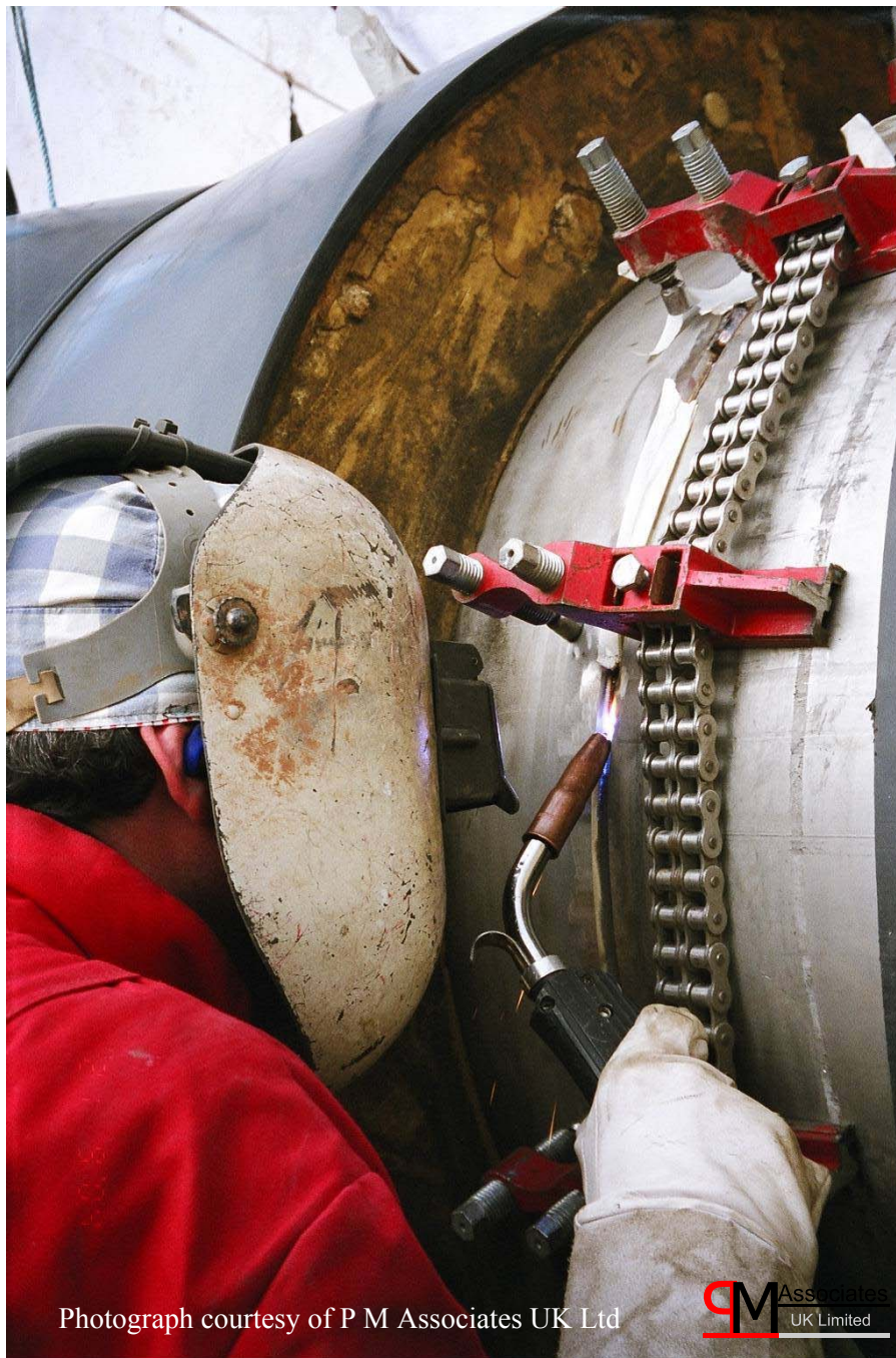
Figure 4 Construction of the Grain-LNG Importation facility on the Isle of Grain, UK; utilising the STT process for the first time in the UK on an LNG plant.
