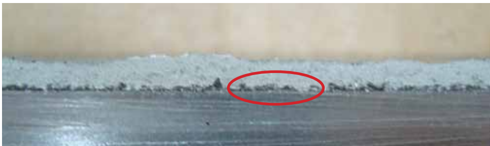
Lack of fusion is evident when the sharp edge of the vertical component can still be seen under the weld metal.
